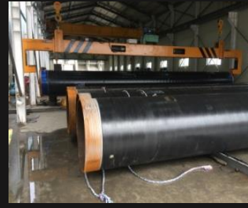
③ Incoming pipe to the shop
